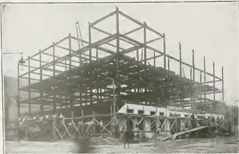
SECURITY BANK BUILDING, MINNEAPOLIS. We are furnishing 1,000 tons of Steel for this Building.
