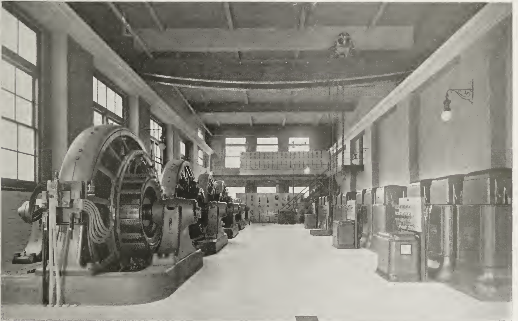
INTERIOR OF ROTARY ROOM AT MINNEAPOLIS SUB-STATION, showing four rotary convertors, units of 3000 H. P. each.
