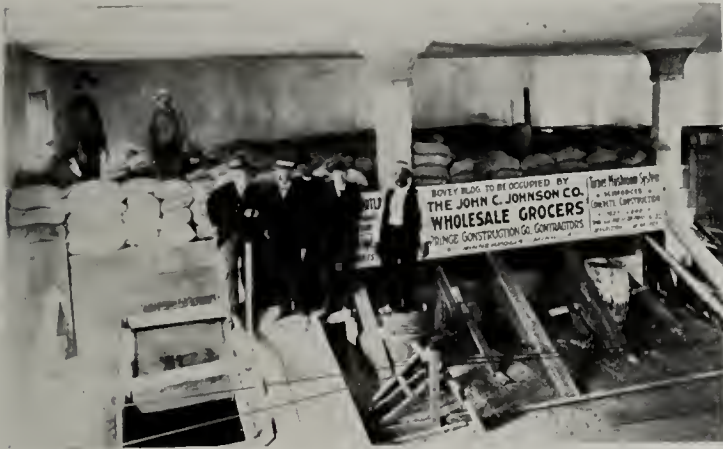
Test load of 180 tons between pannels, applied to Mushroom System. Deflection scant \frac{1}{4} of an inch.
