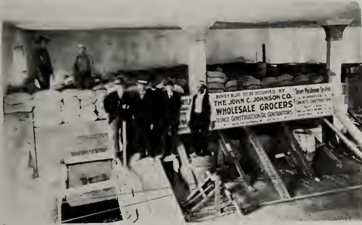
Test load of 180 tons between pannels, applied to Mushroom System. Deflection scant \frac{1}{4} of an inch.
