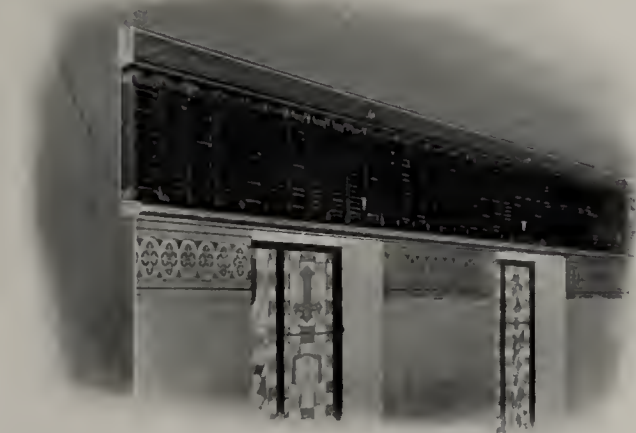
AMERICAN Colonial Wall Radiation as installed and now in use in Epiphany Cathedral, Sioux City, Iowa.
