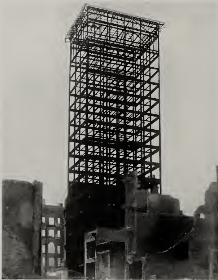
The steel frame and the foundation were well done in the big building
