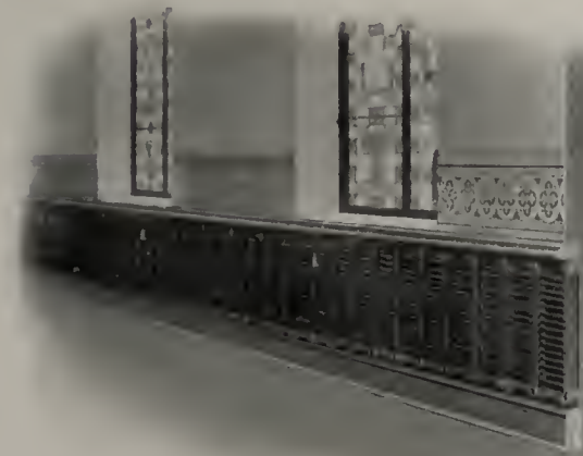
AMERICAN Colonial Wall Radiation as installed and now in use in Epithany Cathedral, Sioux City, Iowa.
