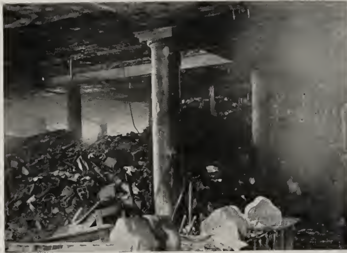
Note load of debris carried on floor; also good condition of remaining arches and column covering.
