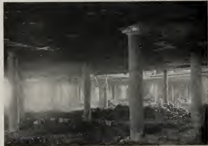
Showing collapse of section of floors caused by failure of column. Note the good condition of remaining floor arches and column covering. If said column had not failed the building would have been practically in perfect condition.
