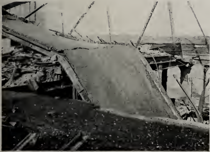
Showing collapse of pent house caused by failure of unprotected steel column. Note reinforced concrete in roof of pent house.
