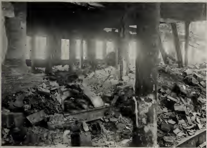
Showing collapse of floors caused by failure of column. Note good condition of remaining arches and column covering.
