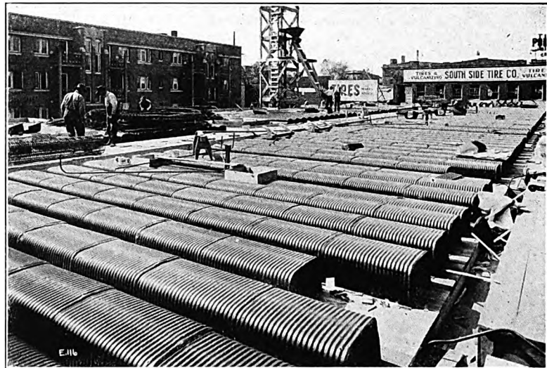
Showing Berger's Pressed Steel Cores installed in the Junius Hotel, Chicago, Ill. Architect: Henry K. Holsman, Chicago
