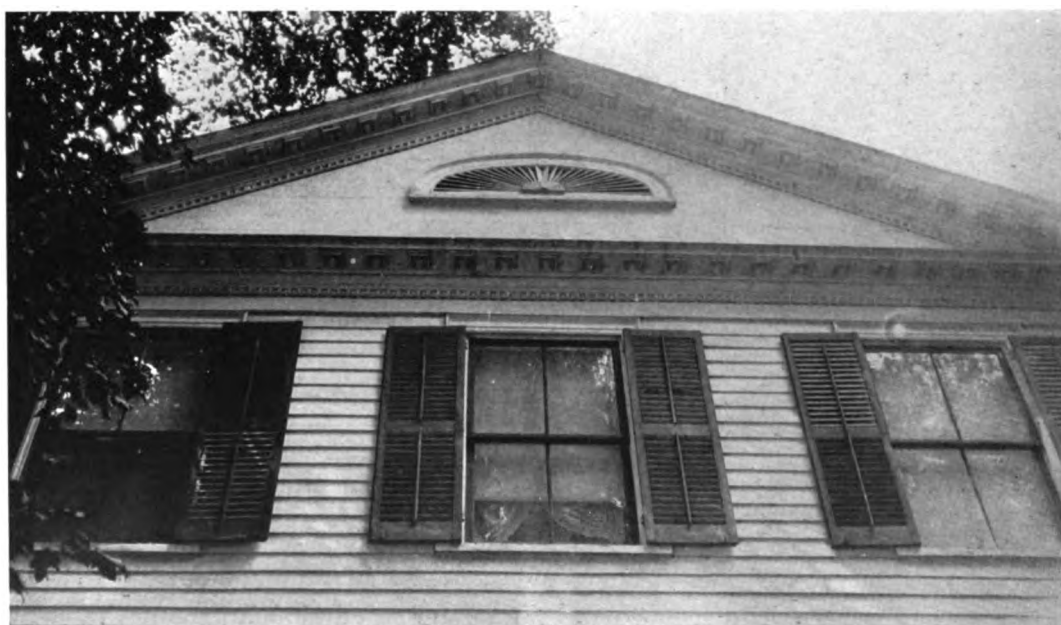
FIGURE 3. DETAIL OF CORNICE OF THE LOCKWOOD HOUSE, MILAN, OHIO. SHOWING THE USE OF HAND MADE, BORED AND GOUGED MOULDINGS AND DETAILS.
