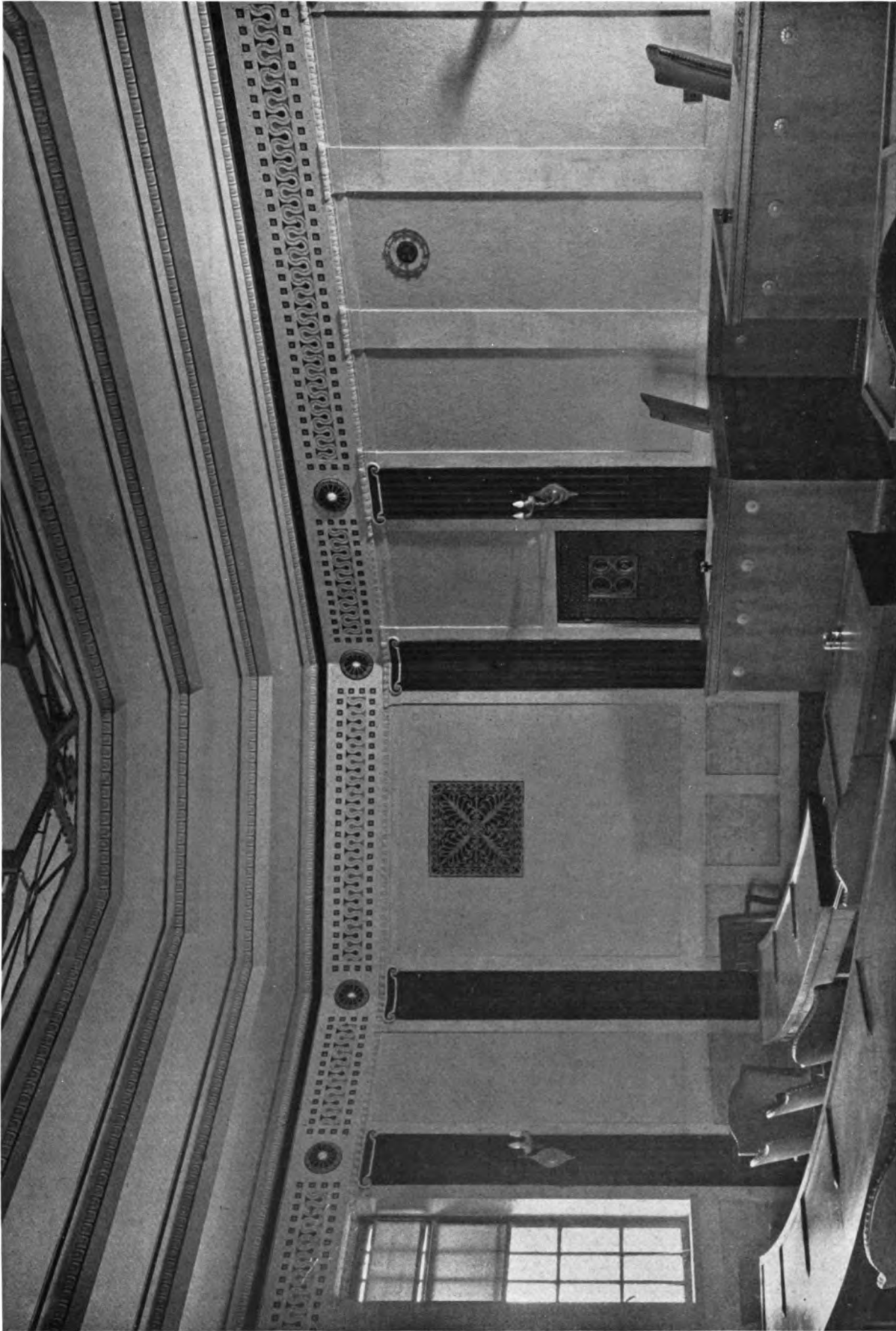
GRAND JURY ROOM COOK COUNTY CRIMINAL COURT HOUSE, CHICAGO ERIC E. HALL, COUNTY ARCHITECT OF HALL, LAWRENCE & RATCLIFFE, INC.
