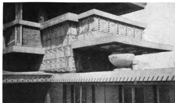
FIG. 5—CONCRETE WALL CAST IN SECTIONS, MIDWAY GARDENS, CHICAGO, ILLINOIS FRANK LLOYD WRIGHT, ARCHITECT
