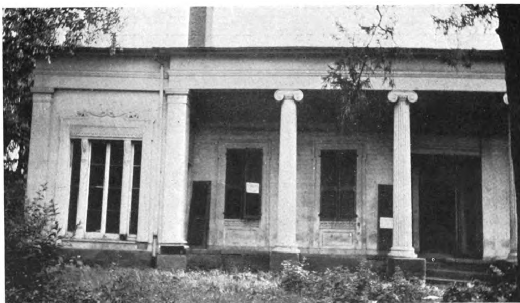
THE JOSEPH SWIFT HOUSE—SHOWING ITS STATE OF DILAPIDATION
