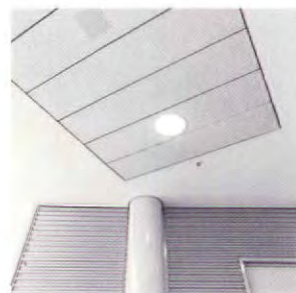
Lufthansa Computer Centre, Frankfurt/Germany
