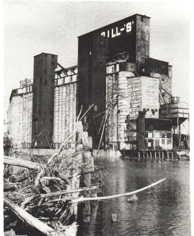
Marine towers and headworks: rusting corrugated-metal cladding visually (but economically!) distinguishes the operational parts of Cargill-Superior elevator from the purely storage volumes in the concrete bins.
