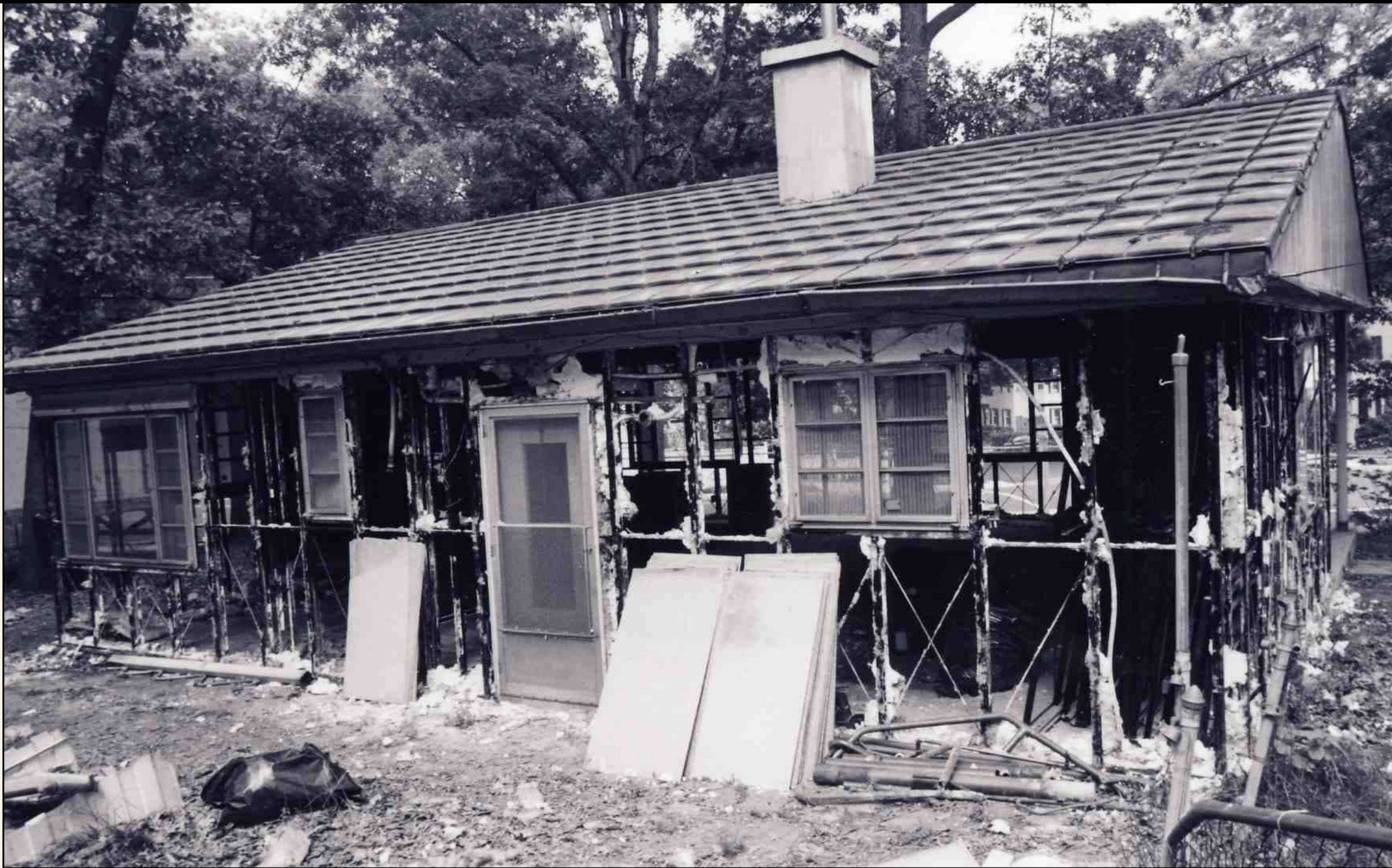
View of rear (west) elevation with all exterior panels and insulation removed. —Victor E. Muncie, May 2006
