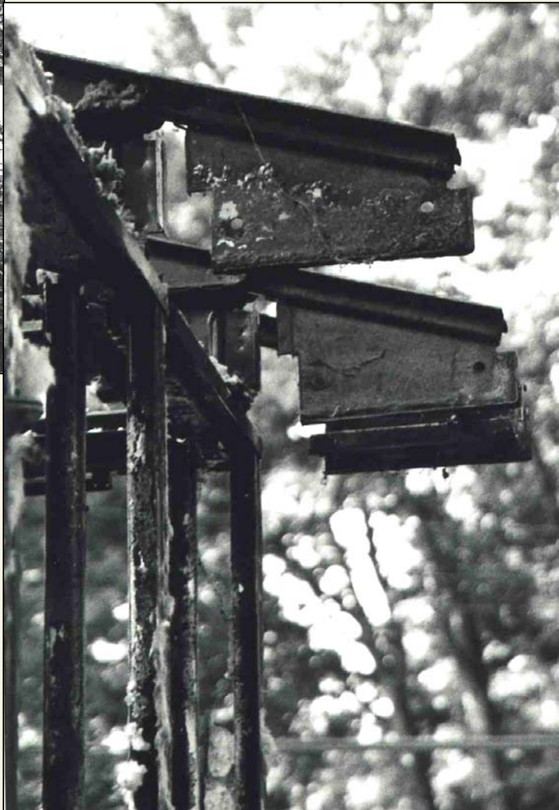
Detail of ends of roof trusses at southwest corner of house. —Cynthia Liccese-Torres, June 6, 2006
