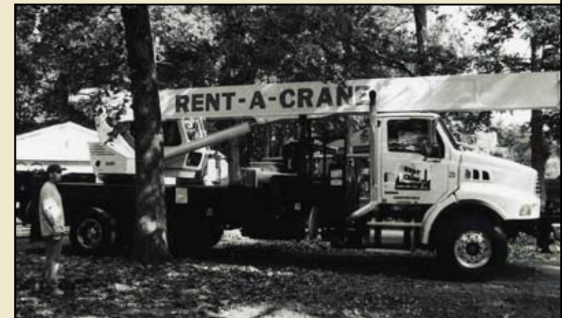
The crane gets situated in the driveway in preparation to remove the roof trusses. —Cynthia Liccese-Torres, June 8, 2006
