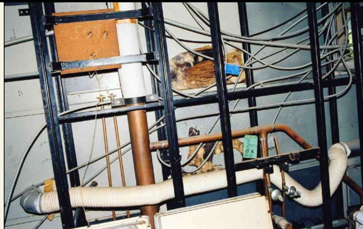
View of original pipes and wiring behind service wall between the bathroom and utility room; note house serial number #549 written in white in upper left and the original green inspection tag from the Lustron factory dated May 9, 1949. —Victor E. Muniec, May 10, 2006
