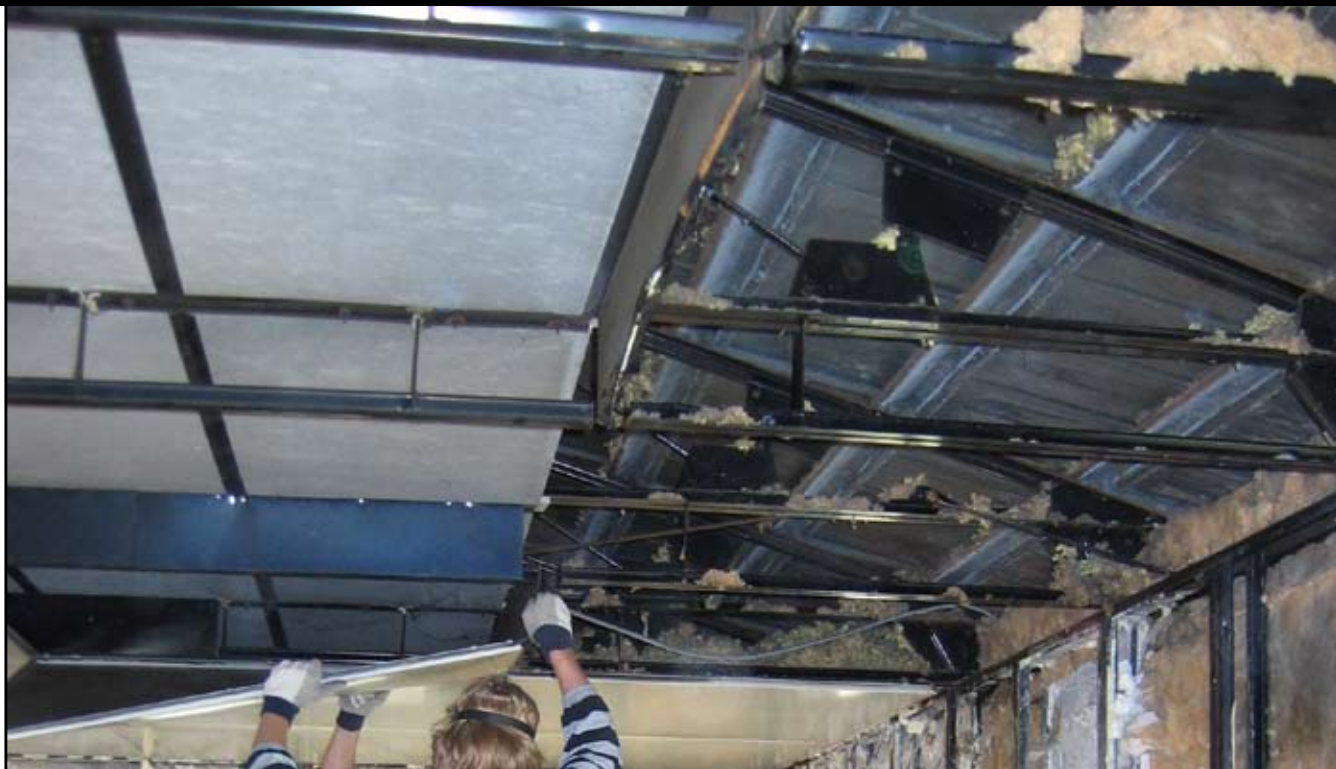
Removal of ceiling panels, looking north towards the master bedroom. —Charles Craig, May 18, 2006
