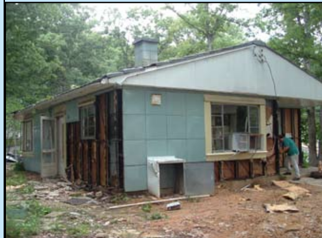
Rear and left side elevations, showing salvaged panels and exposed wall framing. —Cynthia Liccese-Torres, August 10, 2005
