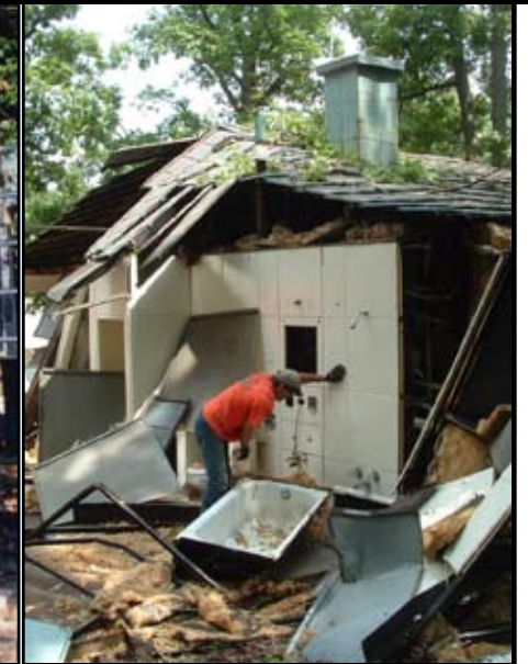
Freeing the bathtub, once the excavator partially demolished the bathroom. —Cynthia Liccese-Torres, August 10, 2005
