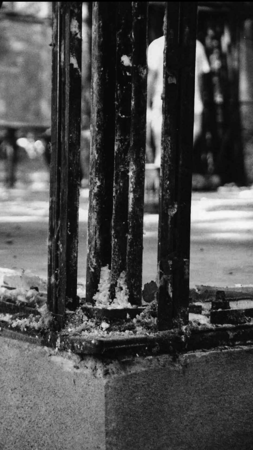
Detail of corner bracing and sill plate; note the large size of the bolt at the bottom right. —Cynthia Liccese-Torres, June 6, 2006
