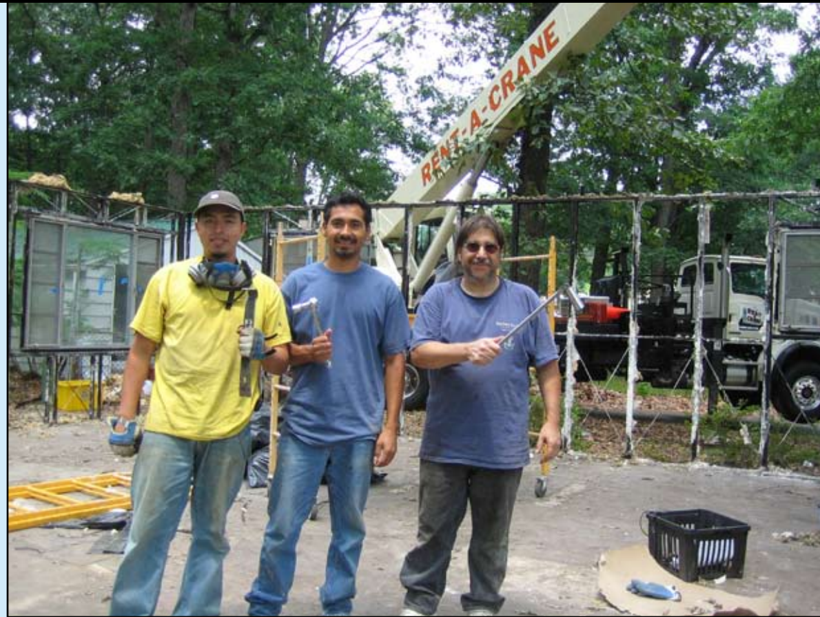
“Have tools, will disassemble.” Crew members prepare for the final hours of the disassembly effort (left to right): Nery DeLeon, David Solis, and Frank Phillips. —Tom Dickinson, June 8, 2006
