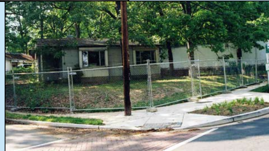
Front (east) elevation just prior to disassembly, with construction fencing around the lot. Note tractor trailer parked in driveway. —Victor E. Muniac, May 3, 2006
