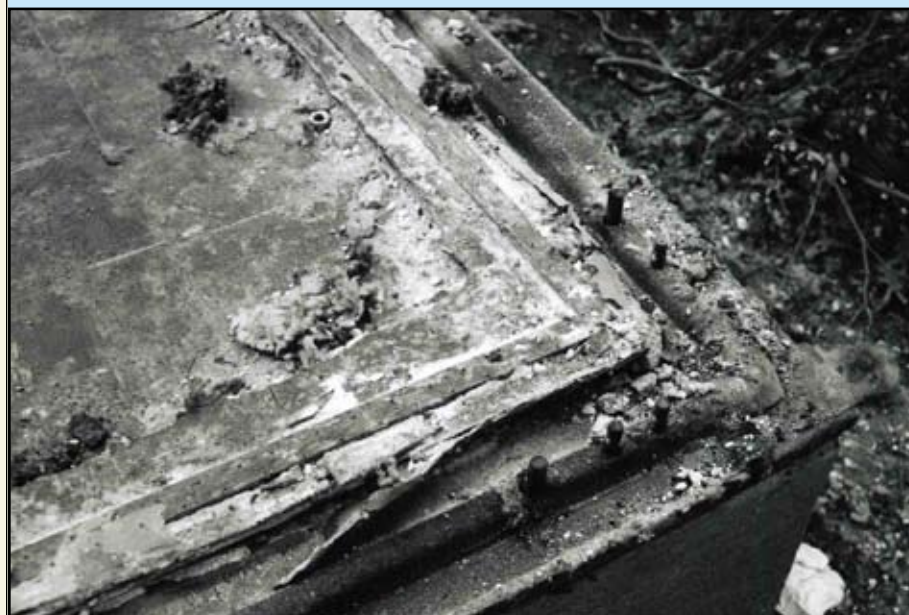
Detail of the metal tracking attached to the perimeter of the foundation where the wall sections were anchored. This tracking could not be salvaged from the Krowne Lustron site. —Cynthia Liccese-Torres, June 8, 2006
