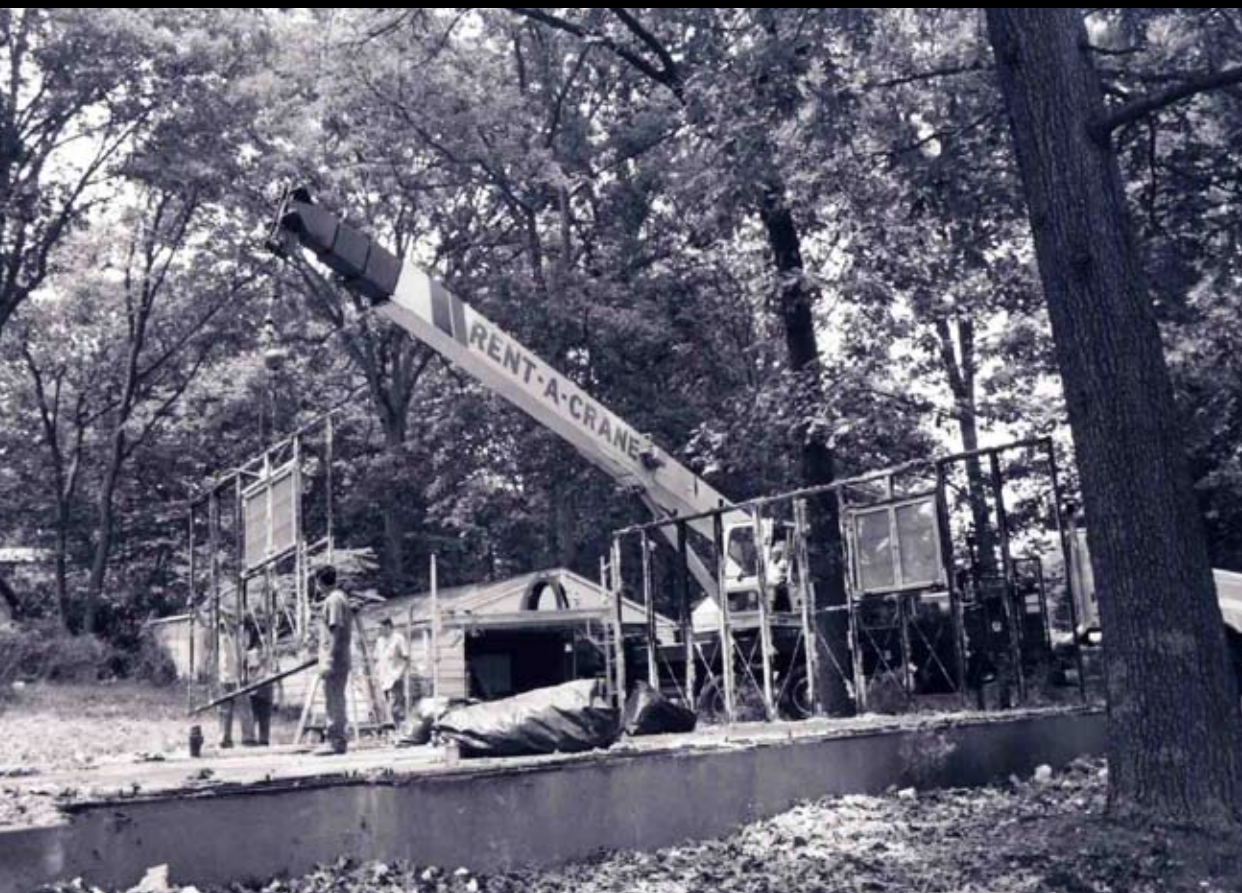
Removal of the first section of the right (north) wall in the rear bedroom. —Victor Muniec, June 8, 2006
