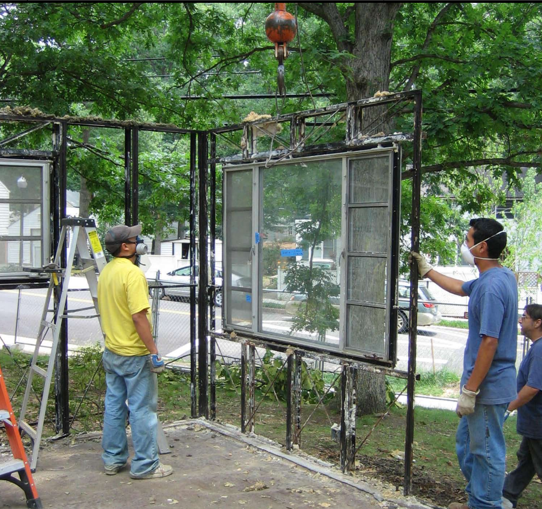
Removal of the wall sections begins; view of the northeastern corner of the house and the master bedroom's front wall. —Tom Dickinson, June 8, 2006
