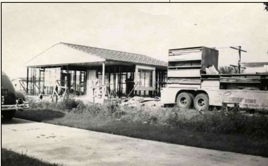
In just two days' time, all the wall framing is up and the roof trusses and panels in place. Image dated June 15, 1949.
