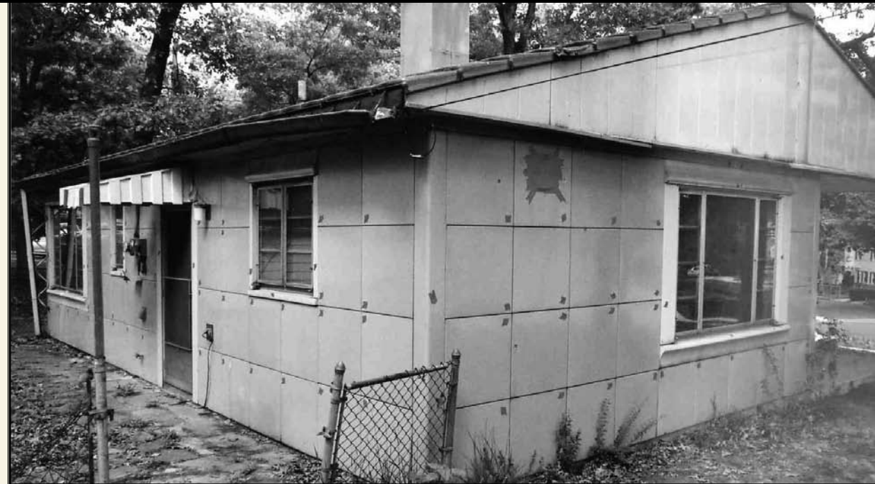
Rear (west) and left (south) elevations, with most exterior panels and features labeled with blue tape. —Victor E. Muniac, May 3, 2006
