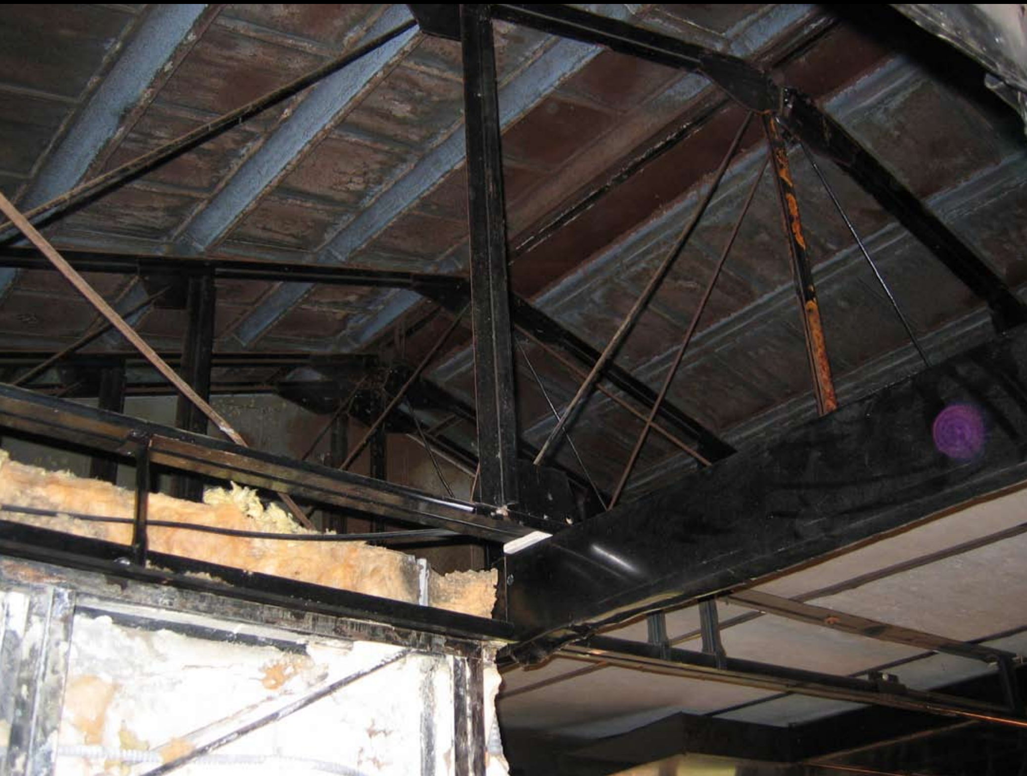
Detail of exposed roof trussing and underside of roof panels. —Charles Craig, May 18, 2006
