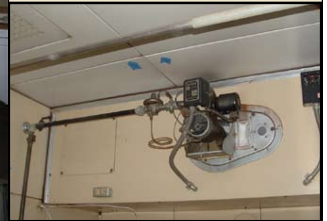
Original and still functional Gas-o-matic furnace surrounded by labeled interior panels. —Marlene Terreros-Oronao, May 3, 2006
