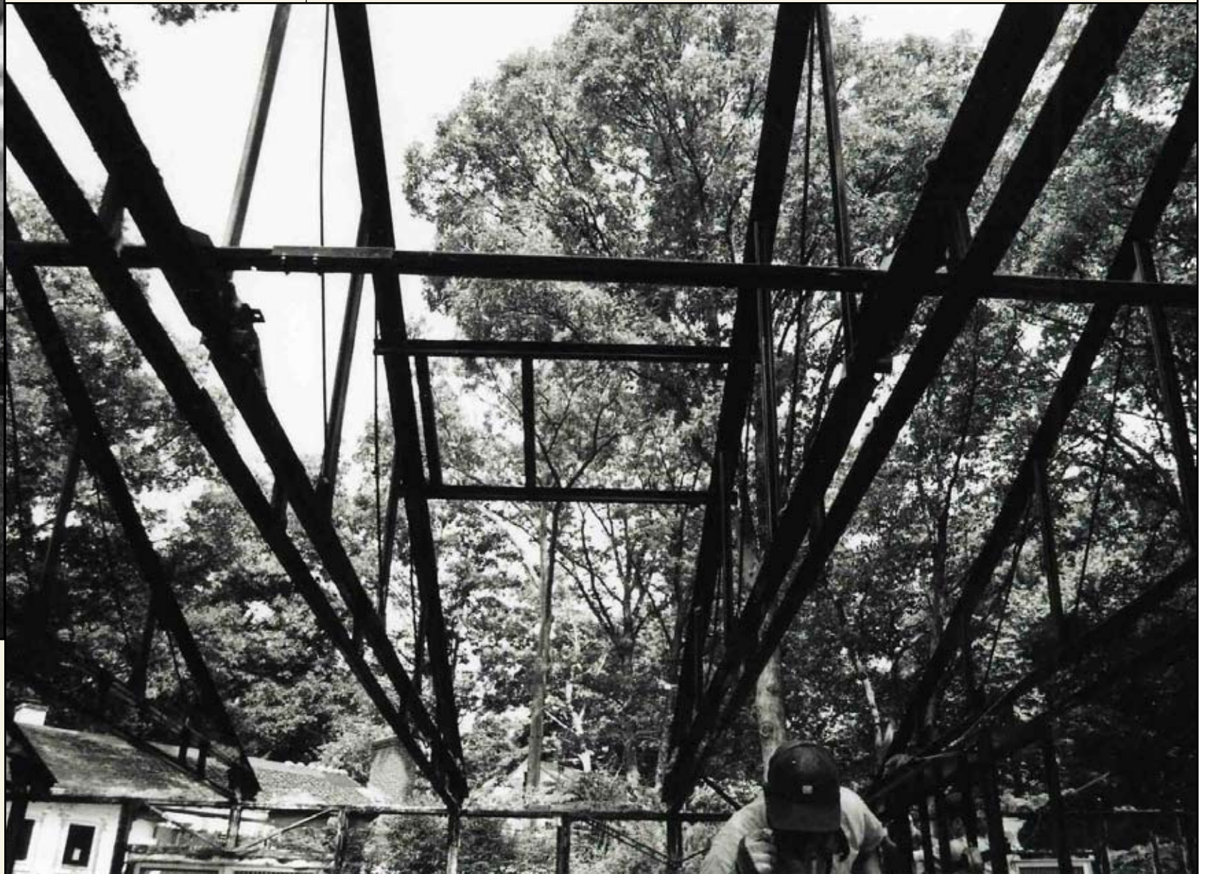
Detail of roof trusses looking up through the roof; note the rectangular opening in the middle for the chimney flue. —Cynthia Liccese-Torres, June 8, 2006
