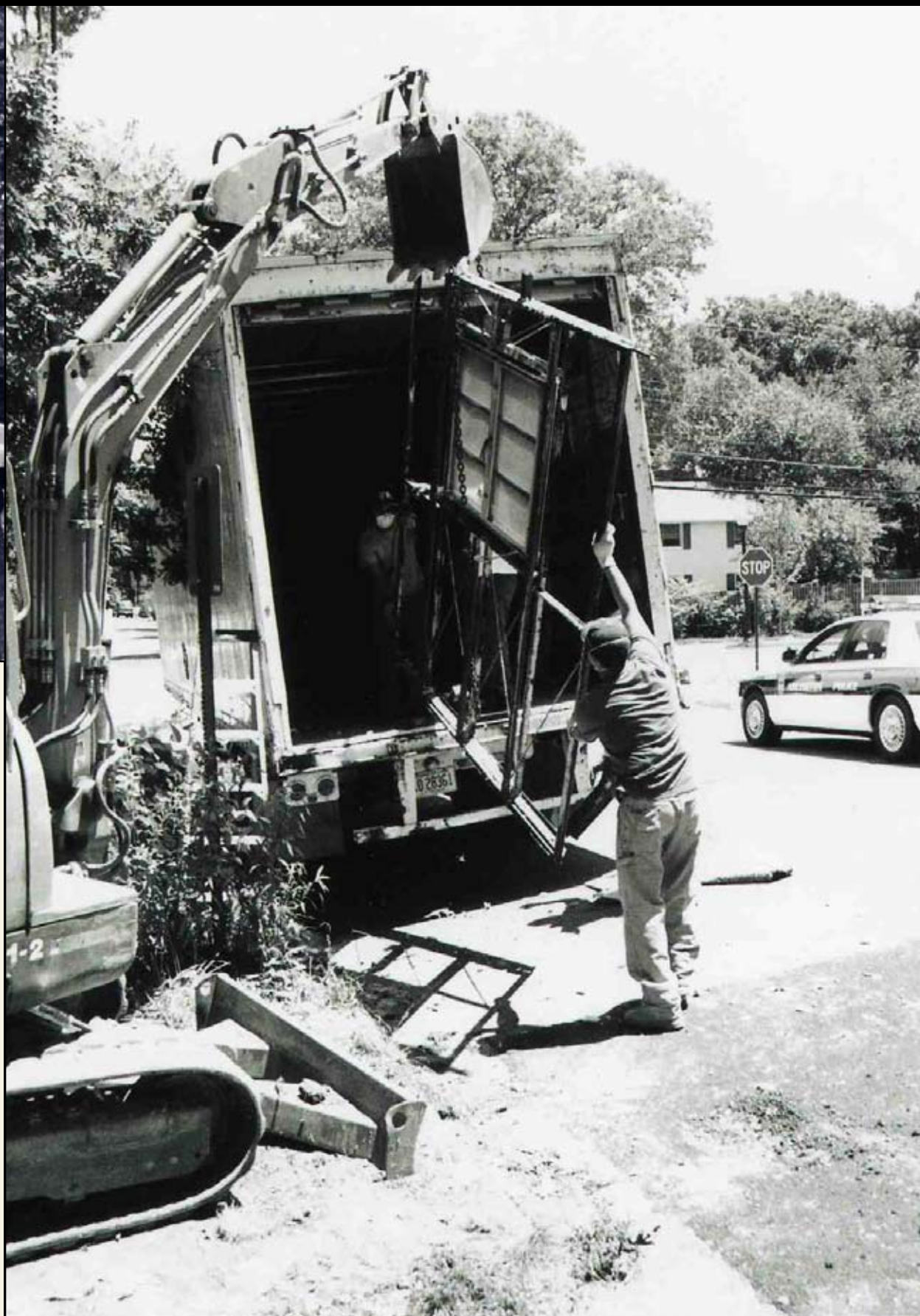
Maneuvering a wall section into the storage trailer with the assistance of a rented Bobcat. —Cynthia Liccese-Torres, June 8, 2006
