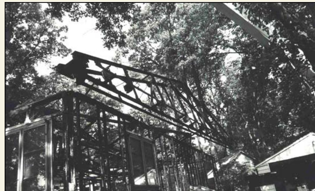
The first roof truss is lifted up and away! —Cynthia Liccese-Torres, June 8, 2006
