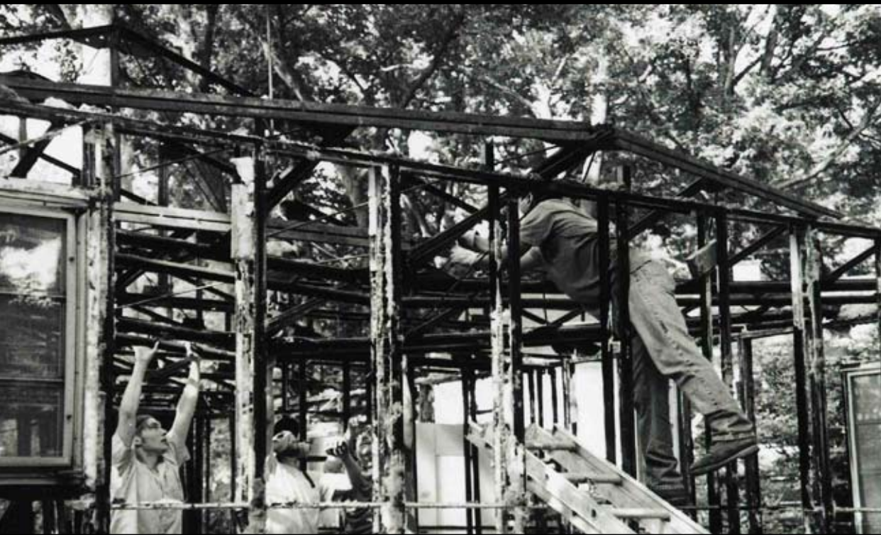
The whole crew adjusts the fallen roof trusses that collapsed upon removal of the first truss. —Cynthia Liccese-Torres, June 8, 2006
