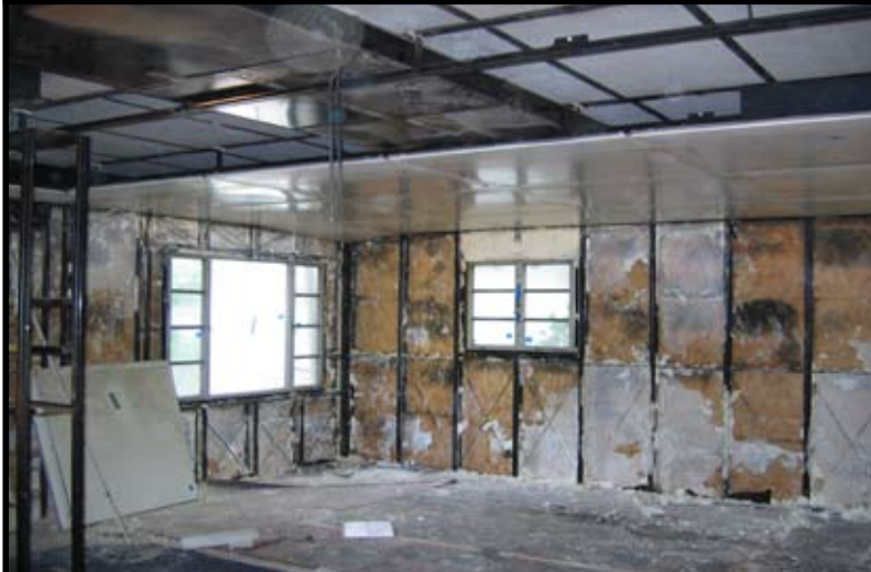
View of second bedroom looking northwest, with exposed wall framing, ceiling panels, plenum, and fiberboard insulating panels above. The plenum is the black rectangular box extending below the insulating panels and above the ceiling panels. —Charles Craig, May 18, 2006
