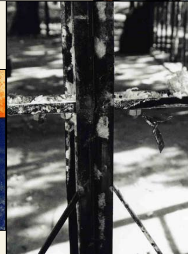
Detail of structural framing with metal tag identifying wall section. —Cynthia Liccese-Torres, June 6, 2006
