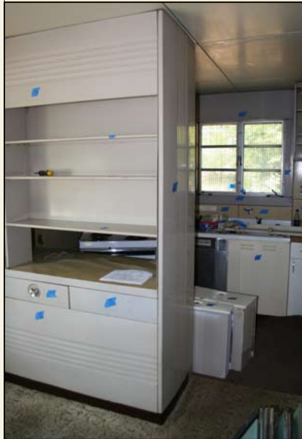
Original dining room china cabinet with pass-through to kitchen, as labeled prior to disassembly. —Todd Zeiger, May 3, 2006
