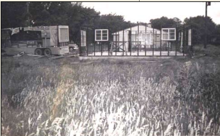
The foundation has set and the wall sections are being installed. Image dated June 13, 1949. In the yard, note the conveniently parked Lustron trailer, which would have been packed in the order needed at the building site. Another Lustron with the small square-shaped bedroom windows, typical of earlier models, already has been completed next door.
