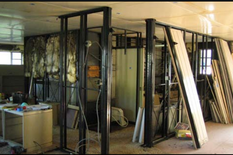
Interior paneling is partially removed, showing the wall sections comprising the bathroom, hallway, and utility room. —Tom Dickinson, May 2006
