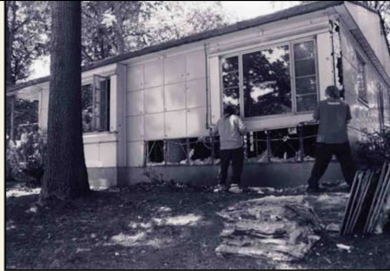
Removal of the first exterior panels on the front elevation; note the pile of fiberglass insulation from the panels stacked on the front lawn. —Victor E. Muniec, May 2006
