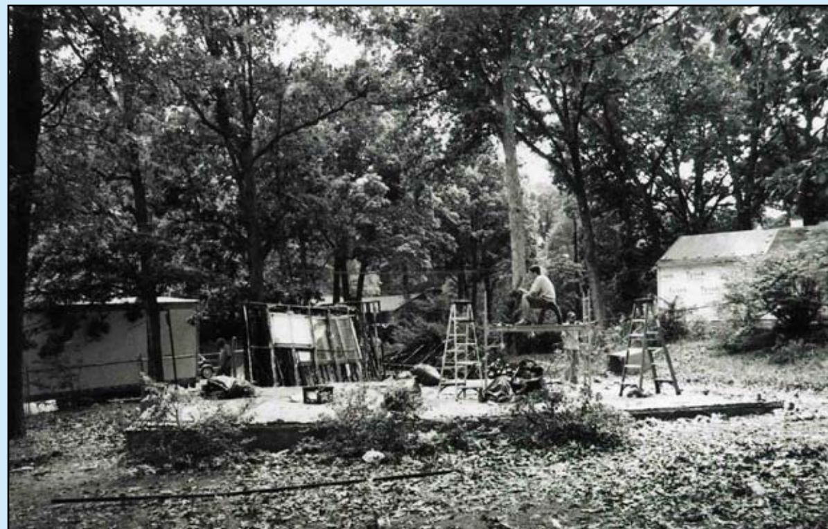
“Hard day’s work.” Only the house foundation and tile flooring remain, as crew member Matthew Phillips reflects on the final day’s progress. —Cynthia Liccese-Torres, June 8, 2006
