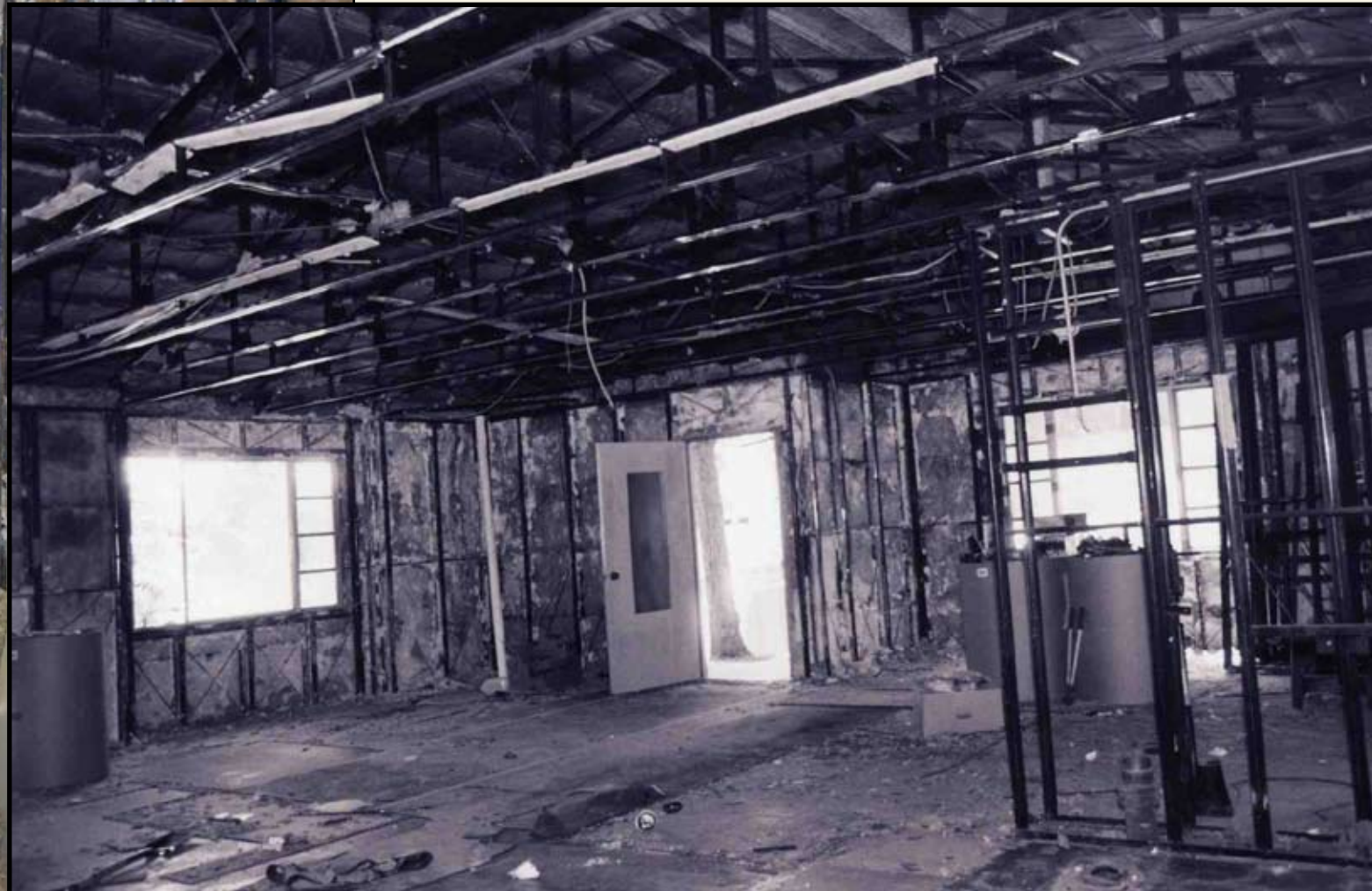
View of gutted interior looking southeast towards the living room. —Victor E. Muniec, May 18, 2006
